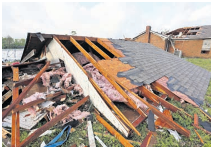
A roof a home that was blown off a home rests on the ground in Hamilton, Miss., after a deadly storm moved through the area Sunday, April 14, 2019.
